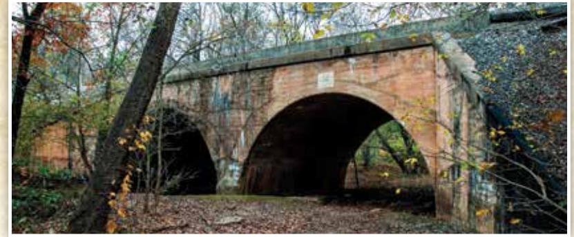
Fig. 5. The Blue Run RR bridge adjacent to Weyburn Road. Blue Run flows under one portal, and Pump House Road used to go under the other. The construction is typical of the early 1900s. Water from the run was pumped the approximate half-mile to the Weyburn coaling station. Photo courtesy of Ann Miller and Zach Barlow.
